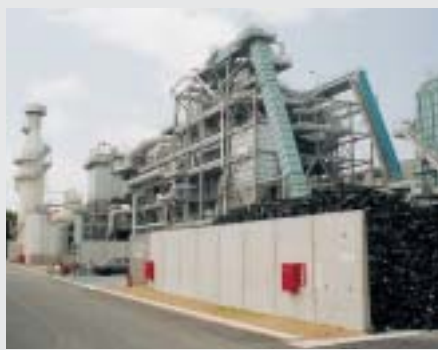
Boiler for waste power generation[*15] will contribute to cost reduction and reducing environmental impact: Nippon Daishowa Paperboard Tohoku Co., Ltd.
