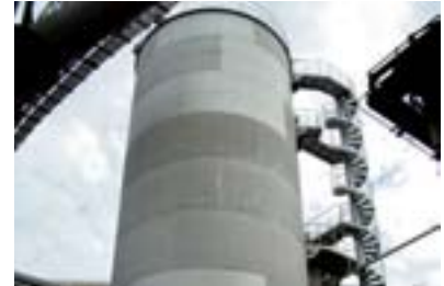
Anaerobic wastewater treatment equipment (Iwakuni Mill of Nippon Paper Industries)
